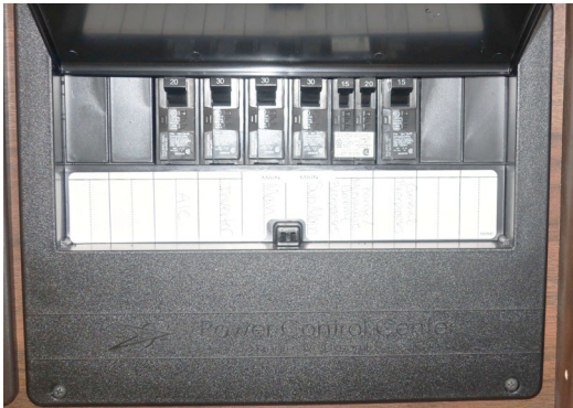
120-Volt Circuit Breakers -Typical View
