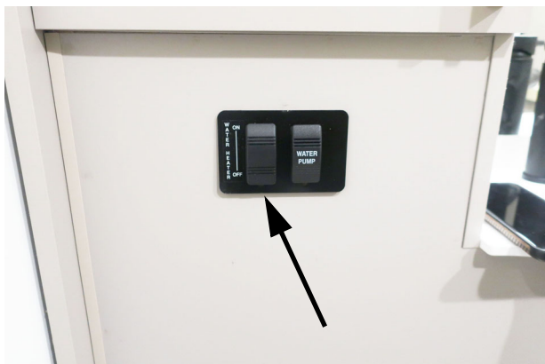
Water Heater ON/OFF switch (Located in the lavatory). -Typical View
