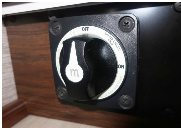
Inverter/charger disconnect switch. (Located inside entrance door next to awning controls -typical view)
