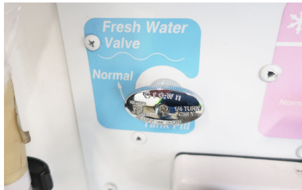
Fresh Water Valve (Located in water service center)
